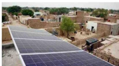
Under the PM Surya Ghar Muft Bijli Yojana, the Centre has already released grants for 1.04 lakh consumers in Rajasthan. FILE PHOTO
