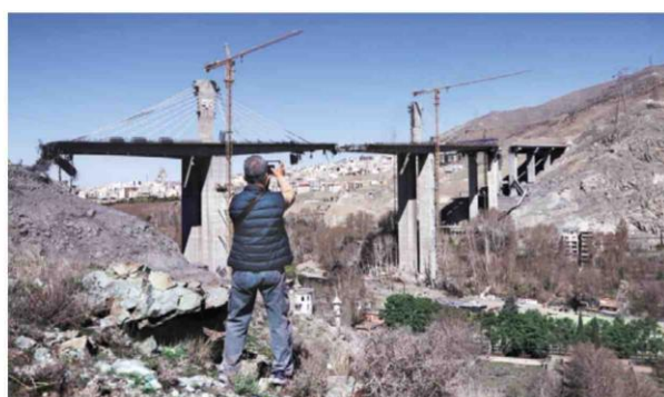
The 136-metre-high B1 bridge in Iran's Karaj has been partially destroyed by joint US-Israeli strikes on Thursday. It is the tallest bridge in West Asia PHOTO: REUTERS
