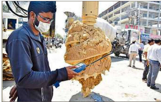
A Gail team inspects leakages near the spot where Metro digging work damaged an underground pipeline. The incident was reported from Garudacharpalya, Whitefield Main Road on October 29.
