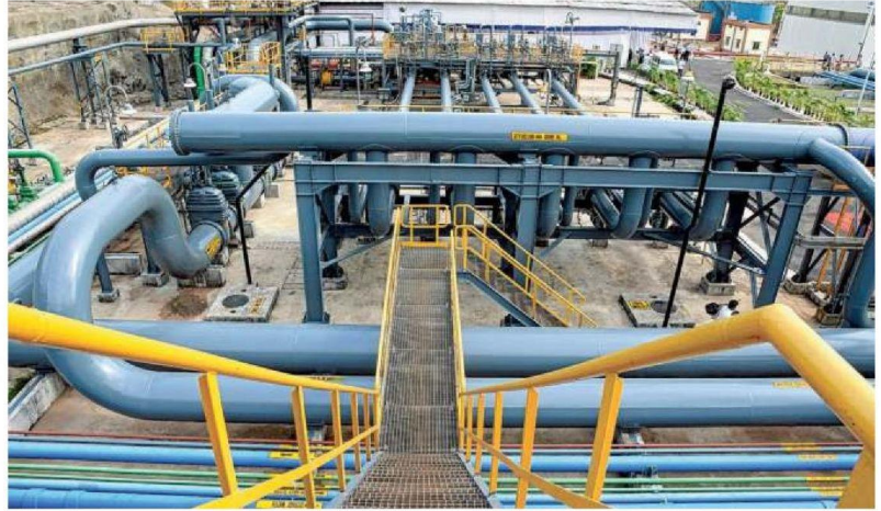
Expansion pipeline A file picture of the Indian Strategic Petroleum Reserves Ltd’s storage unit in Mangaluru MANJUNATH HHS
