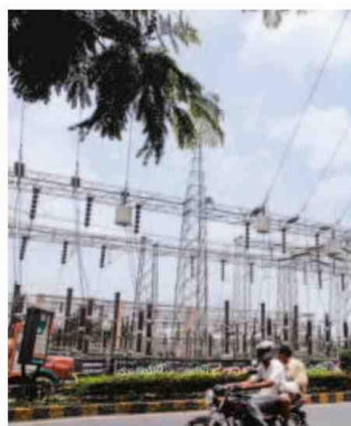
Power cuts were caused by grid tripping, load shedding.
