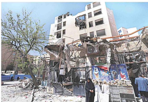
Debris lying in front of a residential building damaged in a US-Israeli strike during the earlier weeks of the war, in Tehran on Tuesday
