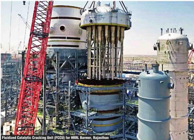
Fluidized Catalytic Cracking Unit (FCCU) for HRRL Barmer, Rajasthan
