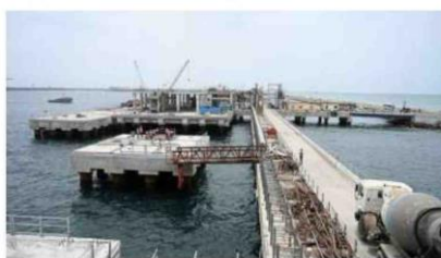
ENHANCING CAPACITY. The jetty will add 3 million tonnes of cargo per annum to the port's capacity. BJOY GHOSH
